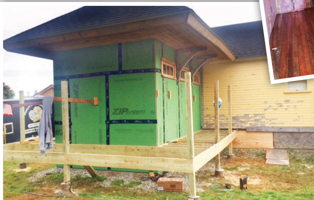
Top: The library now has new steps making for safe entry into the building Middle: Rocky Gould and Steve Canapetti of Rocky's Maintenance installing a wood floor in the library's ell with repurposed wood Bottom: A handicap ramp is also being added to the library
